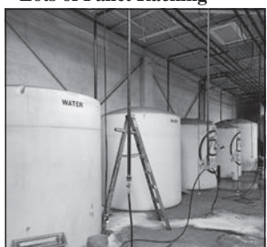
3000 Gallon Water Tanks
